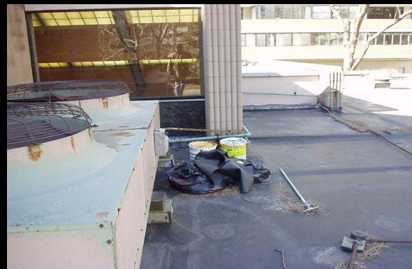
Old chiller/RTU + no insulation
